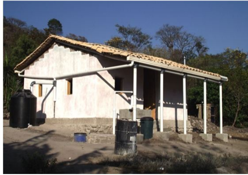
Figure 1: Rainwater tank and hookup.
