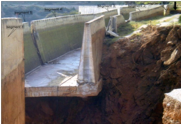
Figure 1: Soil subsidence uphill of the left canal wall between segments 1 and 2 [2].
